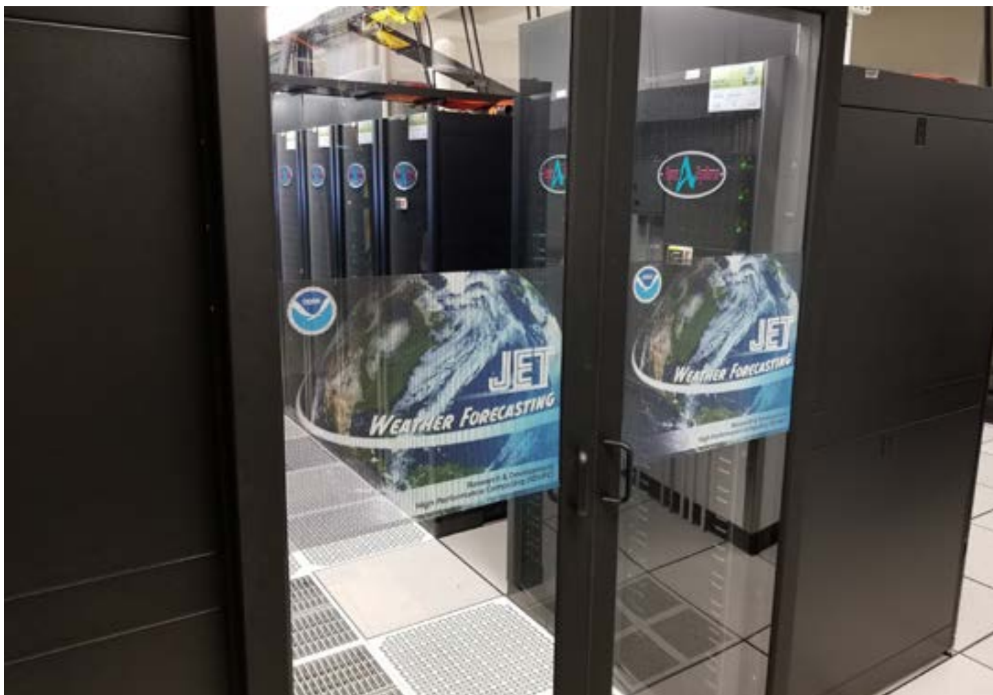
The state-of-the art high-performance computing center, known as JET, at NOAA Boulder.
